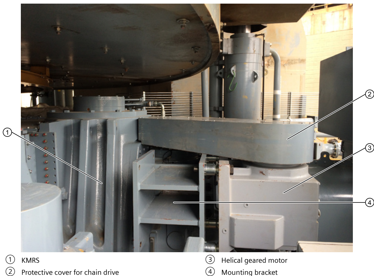
Figure 3-5 Maintenance drive mounted on the KMRS
